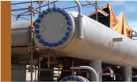
Liquid Outlet Manifold
