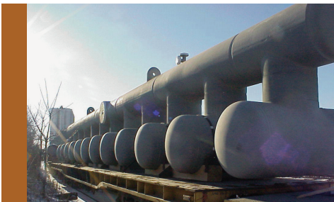
Dry Gas Outlet Manifold
